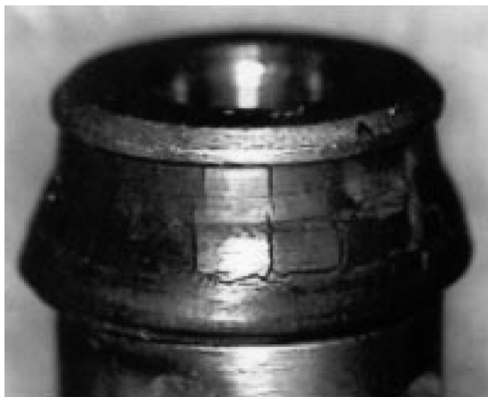
Photo 2 Cracking of check valve seal
